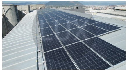
Picture 8. Rooftop solar photovoltaics (PV)
