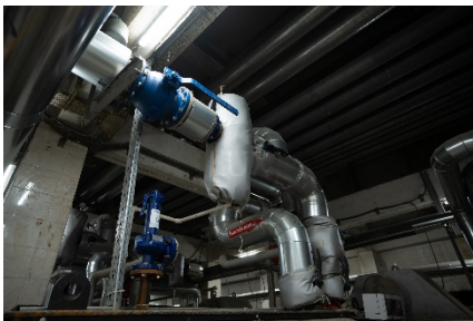
Picture 3. Boiler Room
