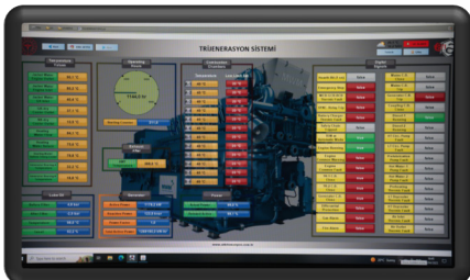
Picture 14. Trigeneration System and Automation Control
