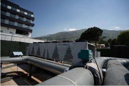
Picture 5. New Variable Speed Air-Cooled Chillers
