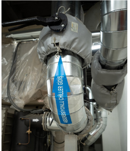
Picture 12. Trigeneneration System and Automation Control
