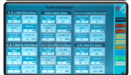
Picture 2. Boiler Room – Boilers, Economizers and Calorimeters
